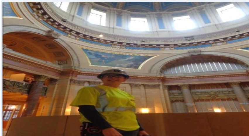
Angela Heikkila, Electrical Foreman for Gephart Electrical, working on the Restoration Project
